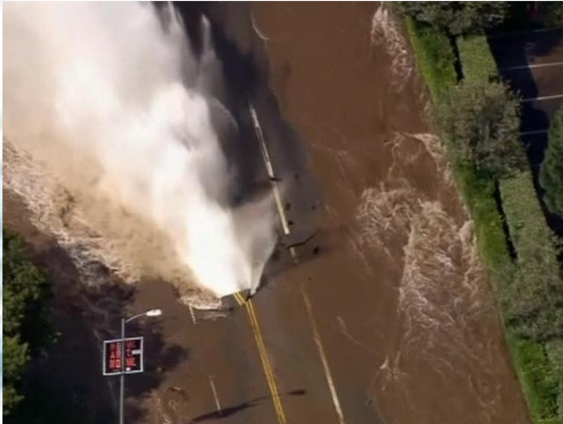
30" water main under Sunset Blvd in California
